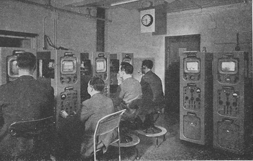
Studio "G" at the Lime Grove Studio Centre, Shepherds Bush, London. The Apparatus Room containing the electronic equipment for the cameras.
