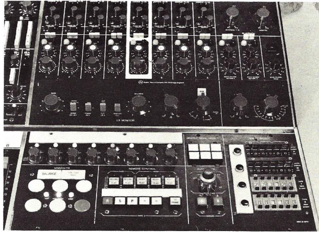
Fig. 4 Part of sound control desk showing, at top, monitoring matrix for MSR, at bottom, remote controls for HVTR and MSR transports, mode and time-code selectors and source switcher.
