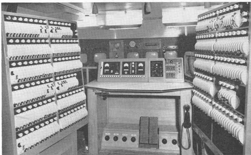
The Lighting Console in the apparatus room of Riverside Studio I. This controls remotely the lighting in the studio and provides 166 control channels each with its own dimmer.
