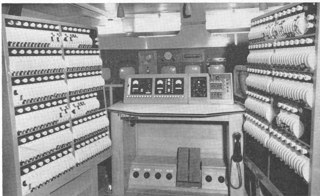
The Lighting Console in the apparatus room of Riverside Studio I. This controls remotely the lighting in the studio and provides 166 control channels each with its own dimmer.
